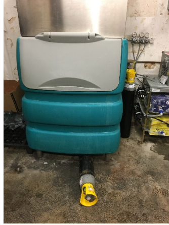
Cellar: CO2 cylinder apparently used to prop up the ice machine.
