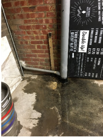
Cellar: Drain pipe has been leaking in the cellar area for some time, but not reported.
