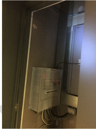
Nightclub area: Open riser is accessed by CSPs (?) to alter lighting rig controls. This is an Estates Riser containing a distribution board. This is an unauthorised use of a high-risk area.
