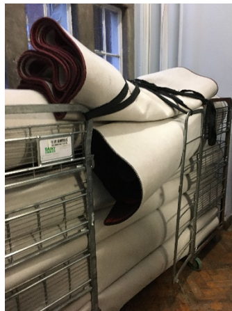
Prayer mats in protected stair well outside kitchen with deep fat fryer with no fire suppression system.
